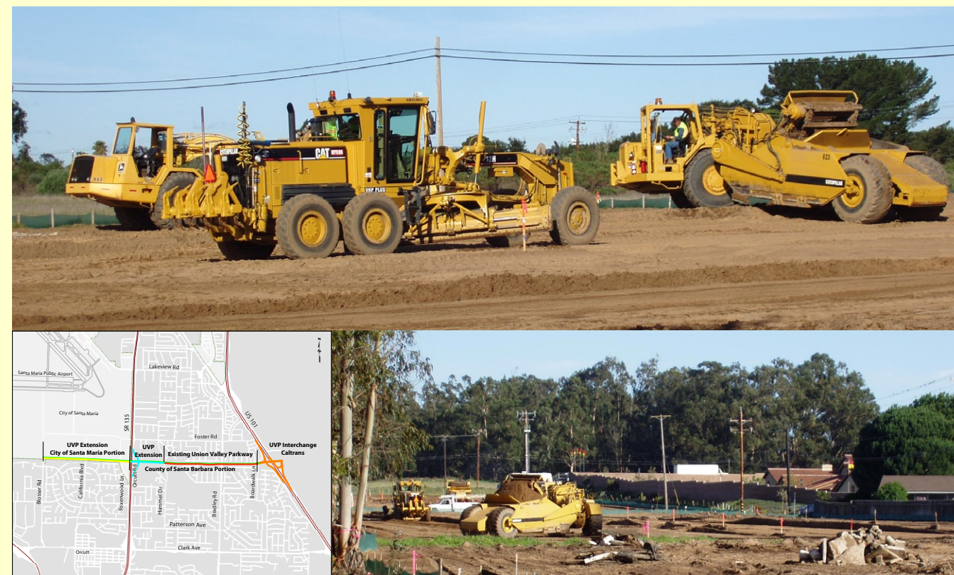
Top: Construction in the City of Santa Maria portion of the Union Valley Parkway Extension in February 2010. In preparation for cleaning out at the end of the day, an elevating wheel tractor-scraper turns around behind a motor scraper between Foxenwood Lane and Highway 135. Bottom left: A map of the UVP project. Bottom right: A view from Santa Barbara County property, west of Foxenwood Lane.
