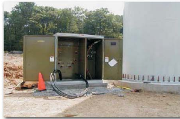
Inset B: Pad transformer beside WTG.
