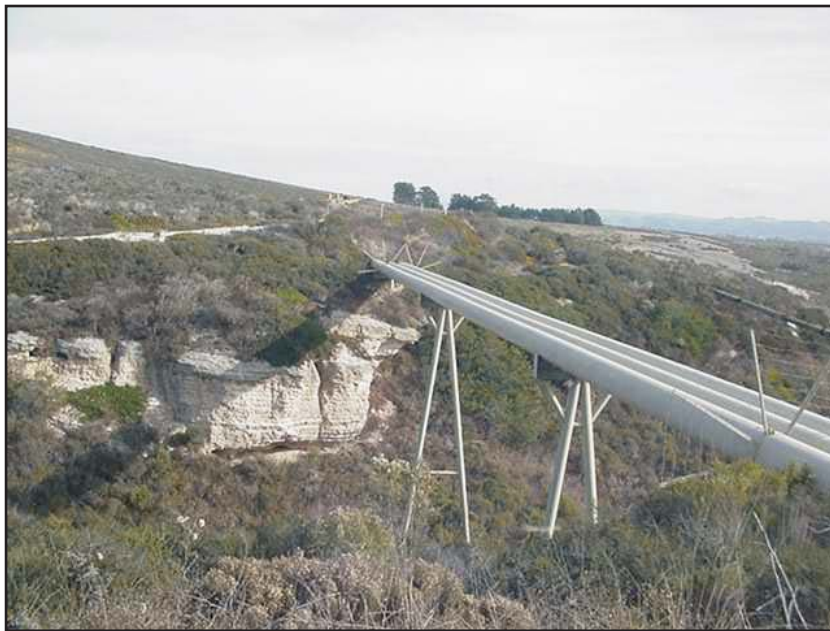
Figures 5.13-8: View of Pipeline Bridge Near Catchment Basin 4 (View Position 7) (Pipelines rack crossing over drainage, view from Terra Road east with the road continuing on the left in the background, three pipelines on the right fore- and mid-ground.)
