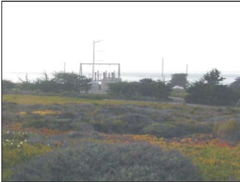
Figures 5.13-3: View of Surf Substation (View Position 2) (View of Surf Substation looking west from the west end of Ocean Avenue. The low vegetation is in the foreground, the substation is in the mid-ground and the ocean is in the background.)
