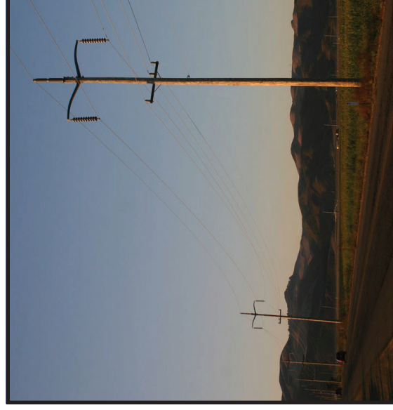
C Example of Typical Power Line Pole Structure
